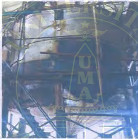
Gambar 3.17 Continous Settling Tank (CST)
