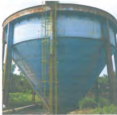
Gambar 3.34 Feed Water Tank
