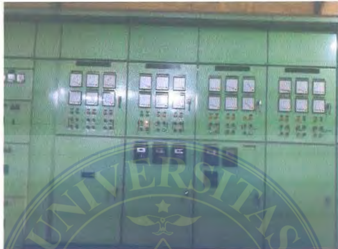
Gambar 3.37 Panel Distribusi Tenaga Listrik
