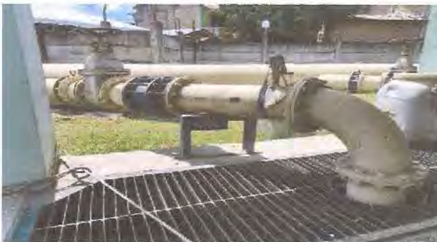
Gambar 3.3 Raw Water Pump
