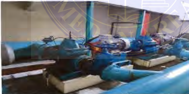
Gambar 3.8 Finish Water Pump
