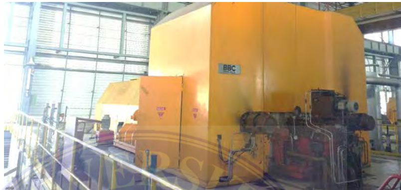
Gambar 2. 4 Steam Turbine PLTU Belawan Unit 3
