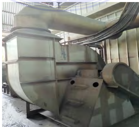
Gambar 2.4 Secondary Air Fan (Sumber: PT Socfindo)
