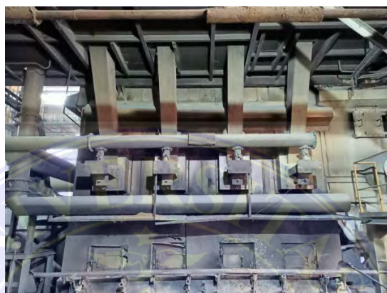
Gambar 2.2 Boiler di PT Socfindo (Sumber: PT Socfindo)
