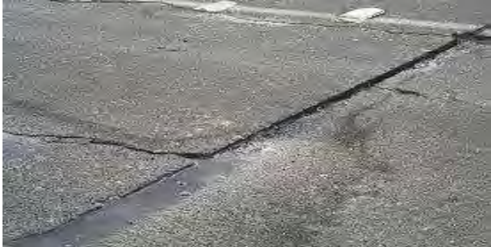
Gambar 4. Patahan ( faulting ) (Nurul Fadillah ,2013)
