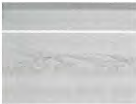
Gambar. 2.3 Retak halus (hair cracks)
