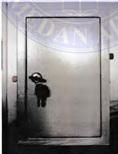
Gambar 3.2(a) panel box solar cell tampak depan
