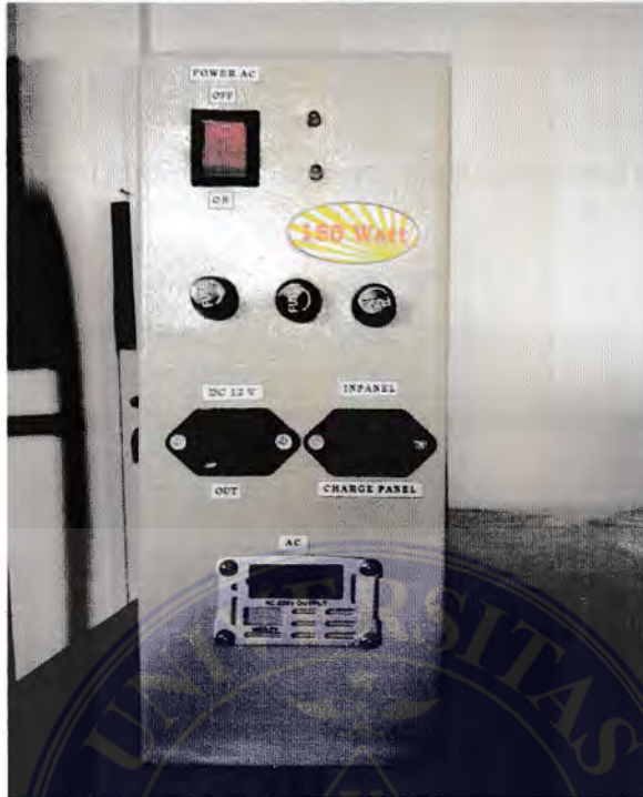
Gambar 3.2 (b) panel box solar cell tampak samping
