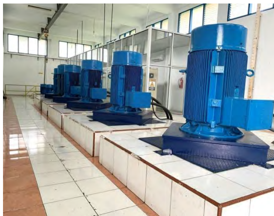
Gambar Finish Water Pump (FWP)
