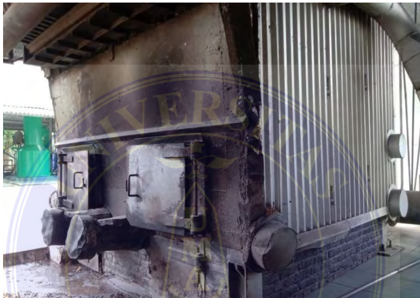
Gambar 3.2 Ruang Bakar Boiler
