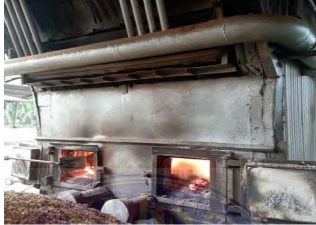
Gambar 2. 9 Ruang Bakar Boiler
