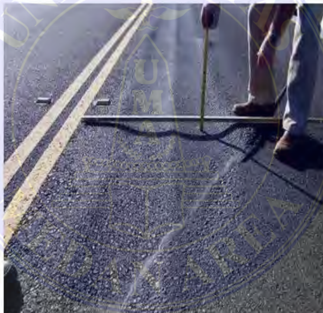
Gambar 5. Kerusakan alur ( rutting ) (Hardiyatmo, 2015).
