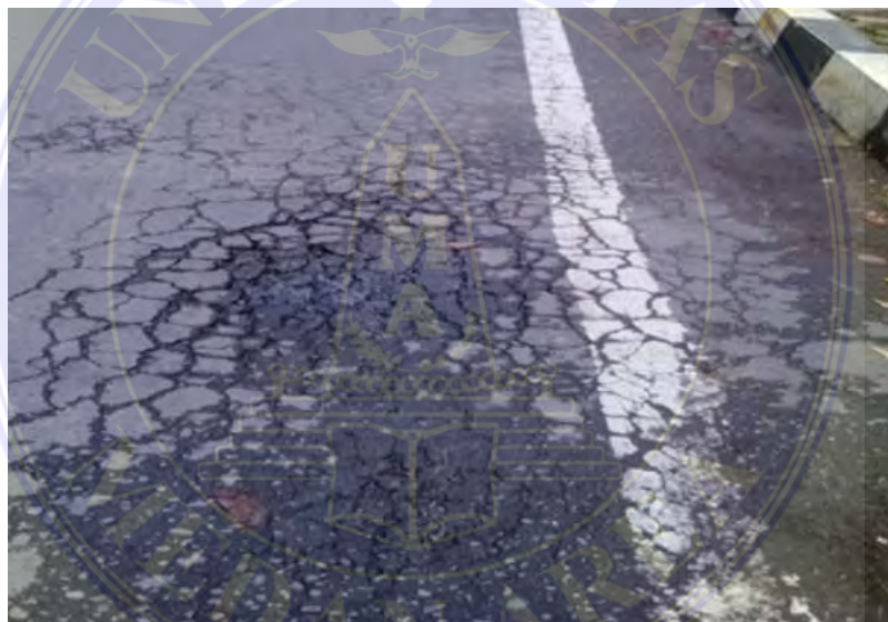
Gambar 33. Kerusakan pinggir/retak pecah ( edge cracks/edge breaks ) (Hardiyatmo, 2015).
