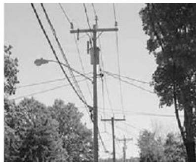
Gambar 2.2 Jaringan Tegangan Menengah ( https://www.slideshare.net/MakmurSaini1/jaringan-tegangan-menengah )
