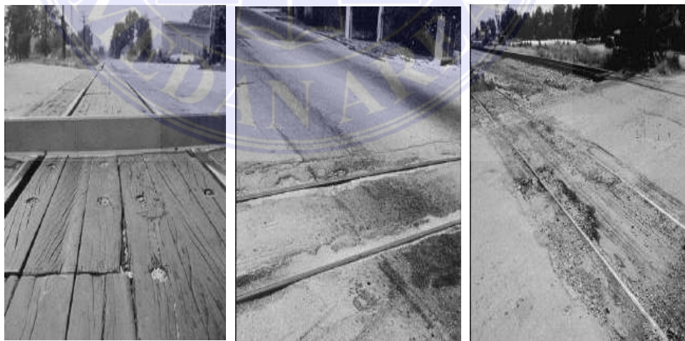
(a) Low (L) (b) Medium (M) (c) High (H) Gambar 17. Rusak Perpotongan Rel ( Railroad Crossing ) (ASTM International, 2018)
