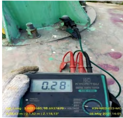
Gambar 3.9: Pengukuran grounding kaki tower 1, pedestal, baseplate dan ankrur condition
