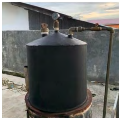
Gambar 2.4 Boiler (Sumber Setiawan et al., 2022)
