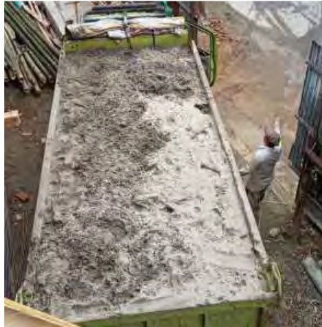
Gambar 3.1.24 Truck Colt Diesel Sumber : Data Lapangan
