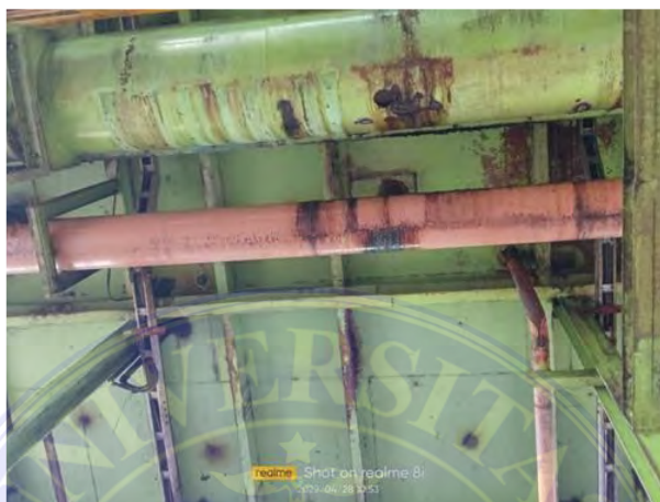
Gambar 3.29. Crude Oil Gutter
