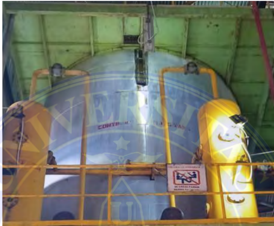
Gambar 3.31. Continious Settling Tank (CST)
