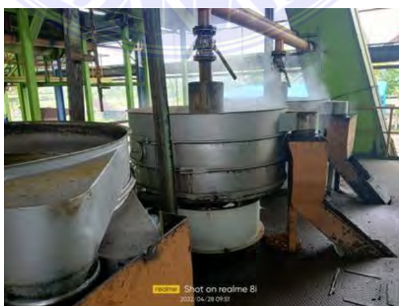
Gambar 3.30. Oil Vibre Separator
