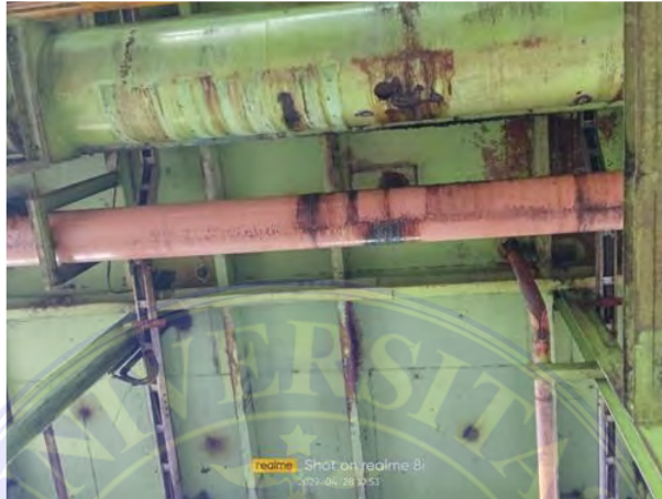
Gambar 3.29. Crude Oil Gutter
