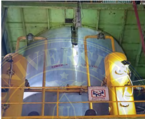
Gambar 3.31. Continious Settling Tank (CST)
