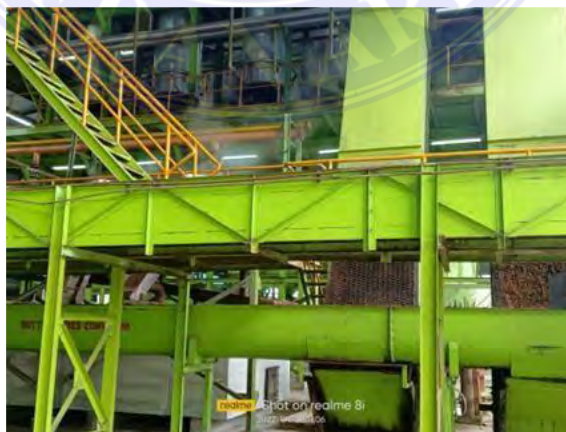
Gambar 3.28. Horizontal Empty Bunch Conveyor
