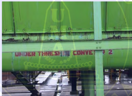
Gambar 3.25. Under Thresher Conveyor
