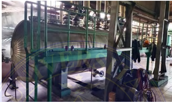
Gambar 3. 32. Back Pressure 3.1.45 Mesin Genset
