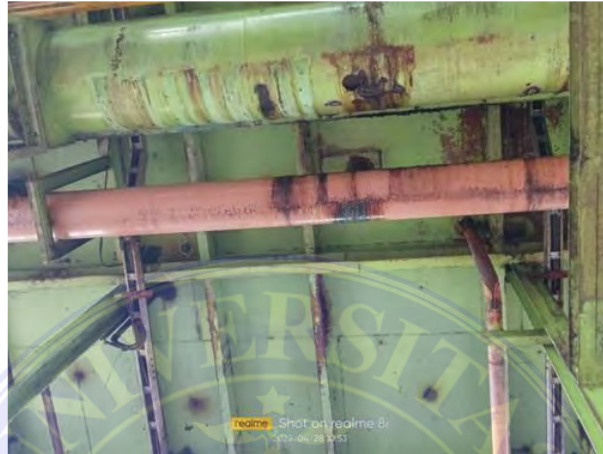
Gambar 3.29. Crude Oil Gutter
