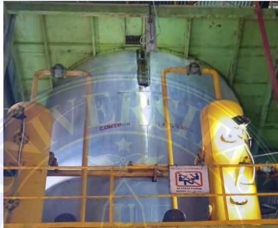
Gambar 3.31. Continious Settling Tank (CST)
