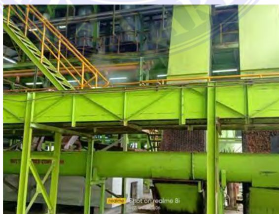
Gambar 3.28. Horizontal Empty Bunch Conveyor
