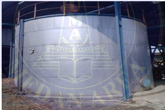
Gambar 3. 53. Feed Water Tank
