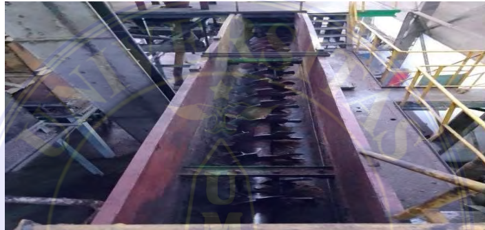
Gambar 3. 22. Cake Breaker Conveyor (CBC)
