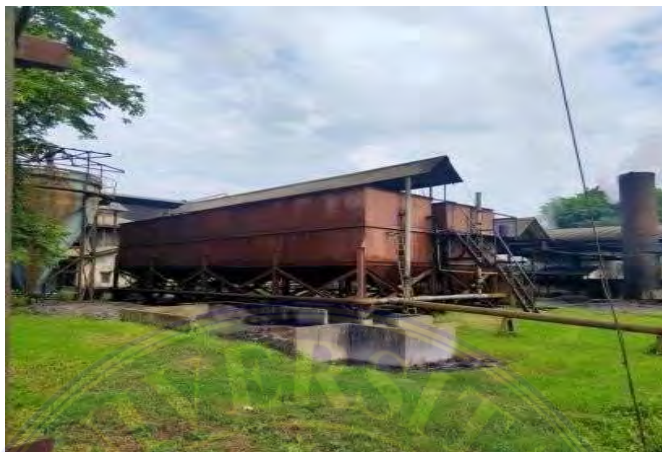
Gambar 3. 58. Bak Recovery Tank
