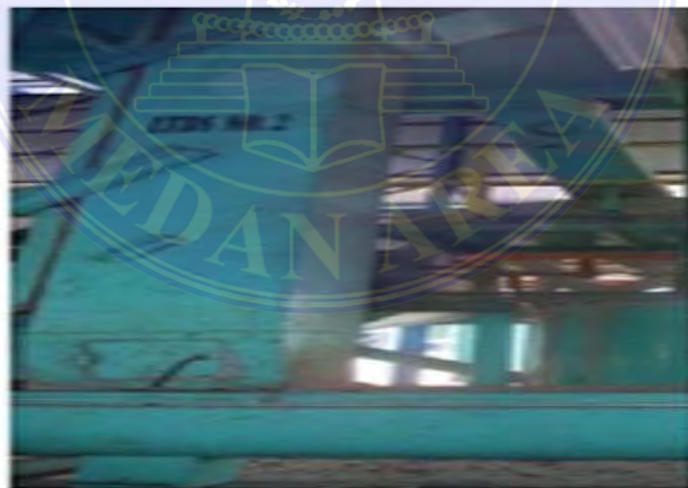
Gambar 3. 41. Cracked Mixture Conveyor
