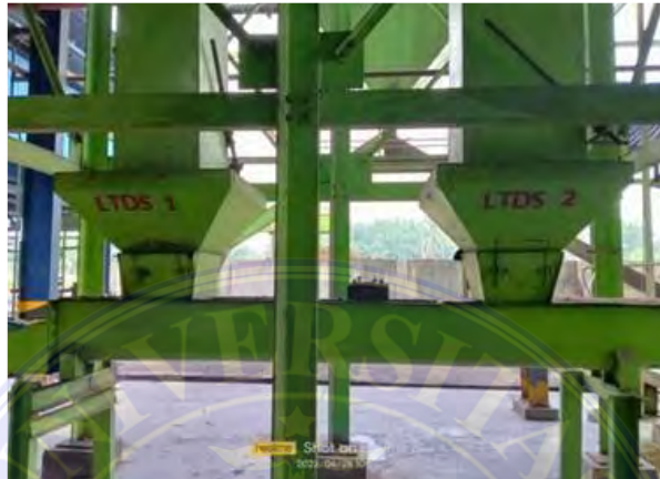
Gambar 3.15. Light Tenera Dry Separator
