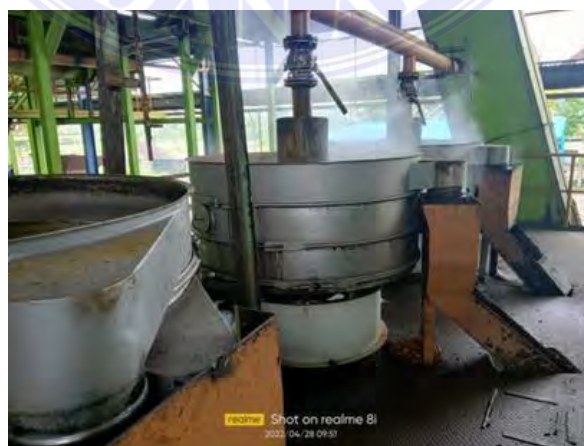
Gambar 3.30. Oil Vibre Separator
