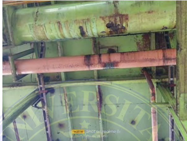
Gambar 3.29. Crude Oil Gutter
