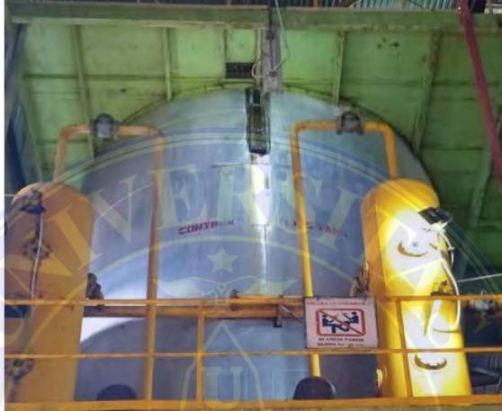
Gambar 3.31. Continious Settling Tank (CST)
