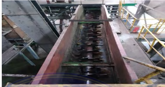
Gambar 3. 23. Cake Breaker Conveyor (CBC)
