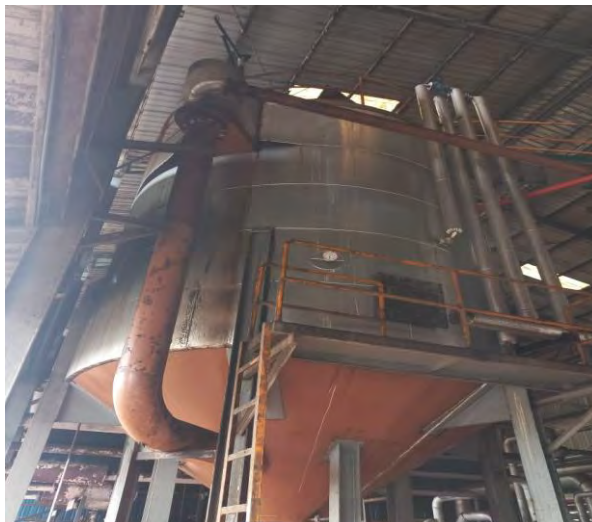
Gambar 3. 15. Continous Settling Tank (CST)
