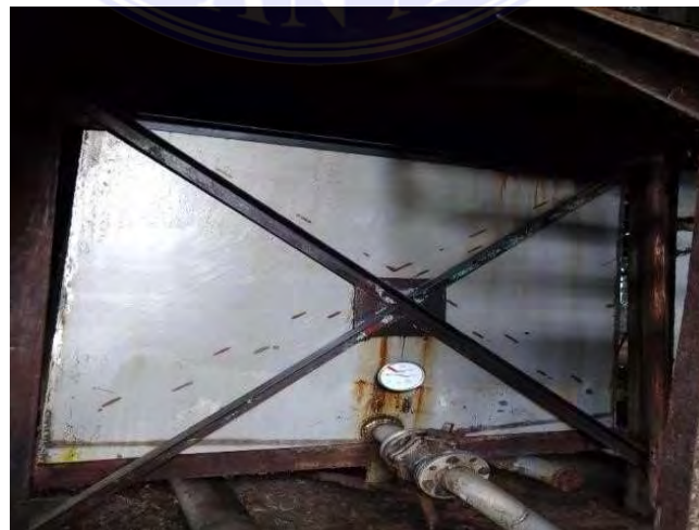
Gambar 3. 25. Crude Oil Tank
