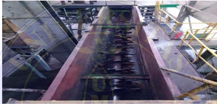
Gambar 3. 22. Cake Breaker Conveyor (CBC)
