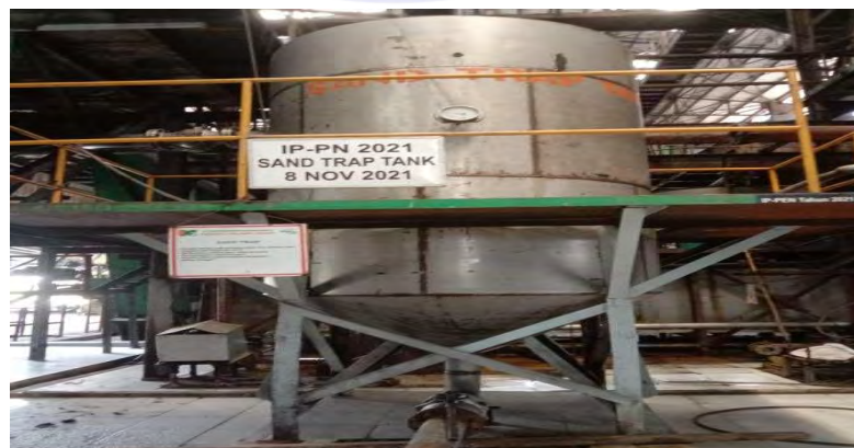
Gambar 3. 23. Sand Trap Tank
