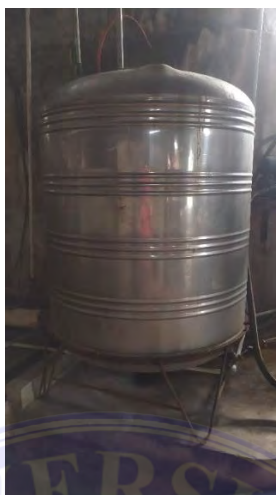
Gambar 3. 9. Feed Water Tank
