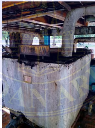
Gambar 3. 19 Crude Oil Tank
