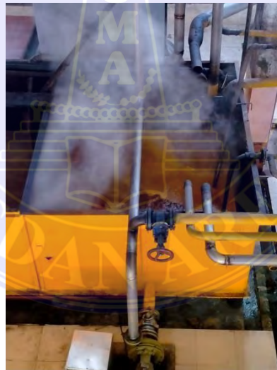
Gambar 3. 26 Oil Collecting Tank
