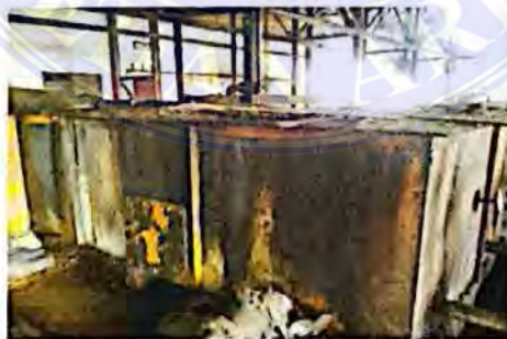
Gambar 3.13. Crude Oil Tank
