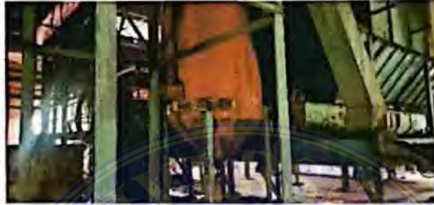
Gambar 3.11. Sand Trap Tank
