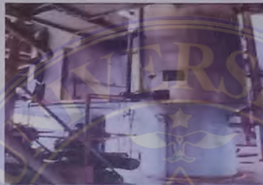
Gambar 3.36. Clean oil tank
