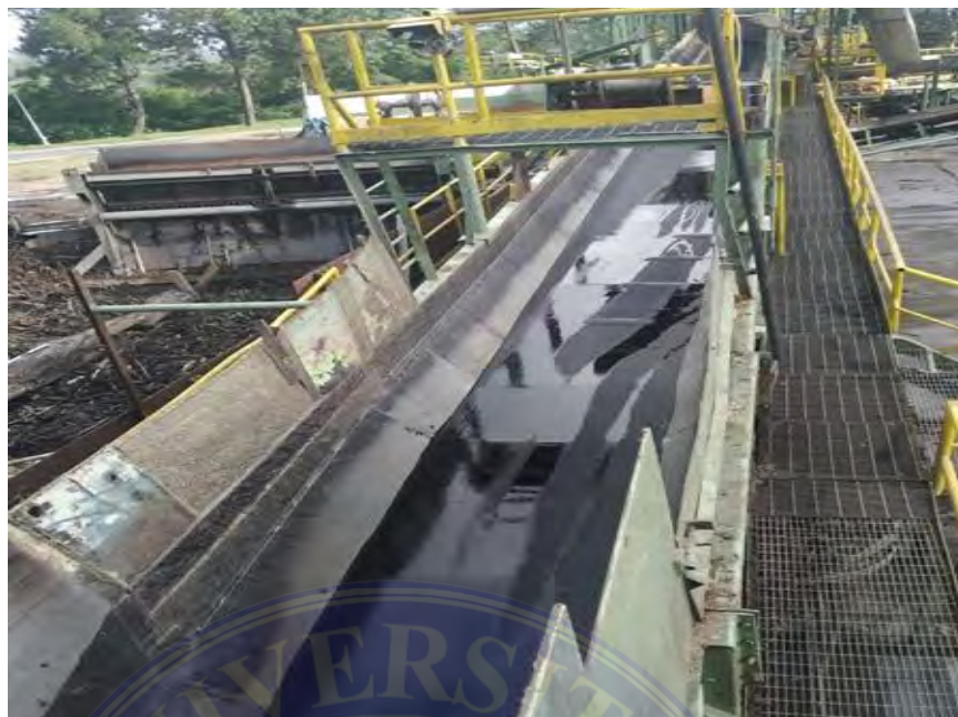
Gambar 3.14. Long Log Belt Conveyor
