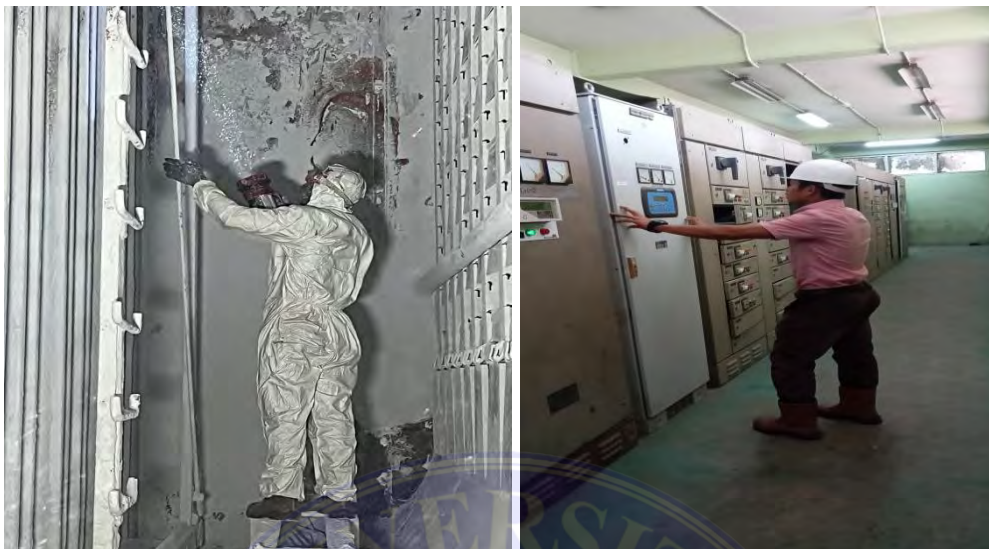
Lampiran 1. Gambar pengecekan Eletroda dan colecting ESP Dan panel ESP
