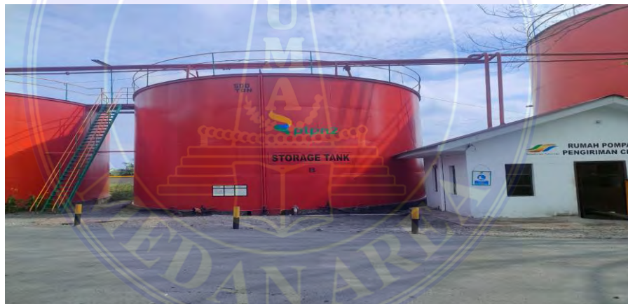
Gambar 3.21. Oil Storage Tank
