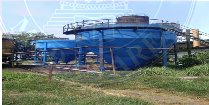
Gambar 3.24. Tangki Pengendapan ( Clarifier Tank )
