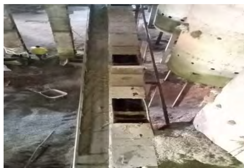
Gambar 3. 22 Cake Breaker Conveyor (CBC).
