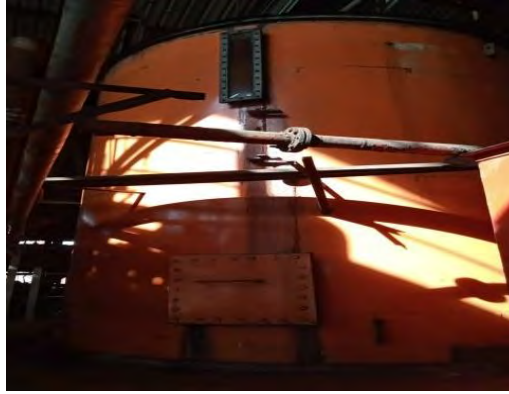
Gambar 3. 15 Continous Setting Tank (CST)
