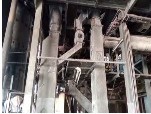
Gambar 3. 28 Light Tenaer Dust Separation (LTDS 1 LTDS 2)
