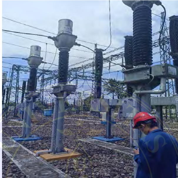
Gambar 3.5 Potensial transformer (PT)
