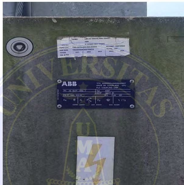
Gambar 4.5 Potensial Transformer (PT)
