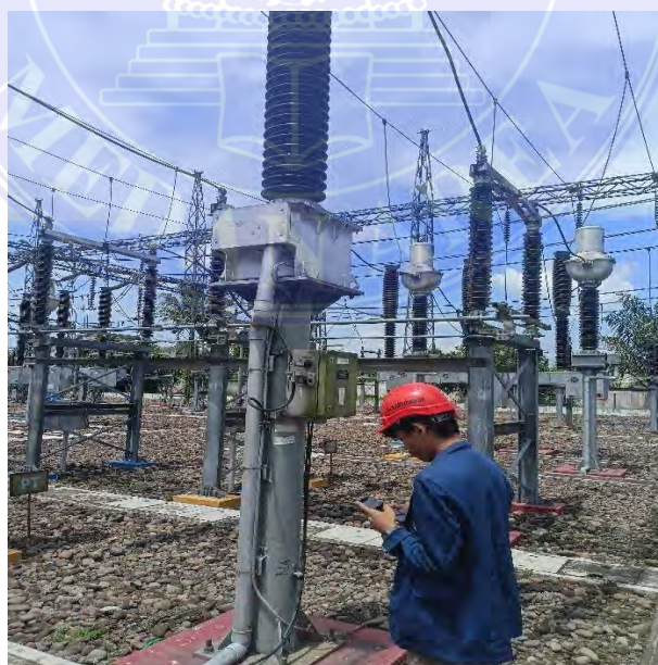
Gambar 3.4 Current transformer (CT)
