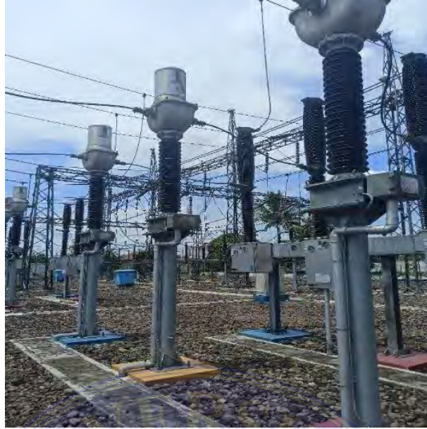
Gambar 2.5 Trafo Tegangan (Potensial Transformer)
