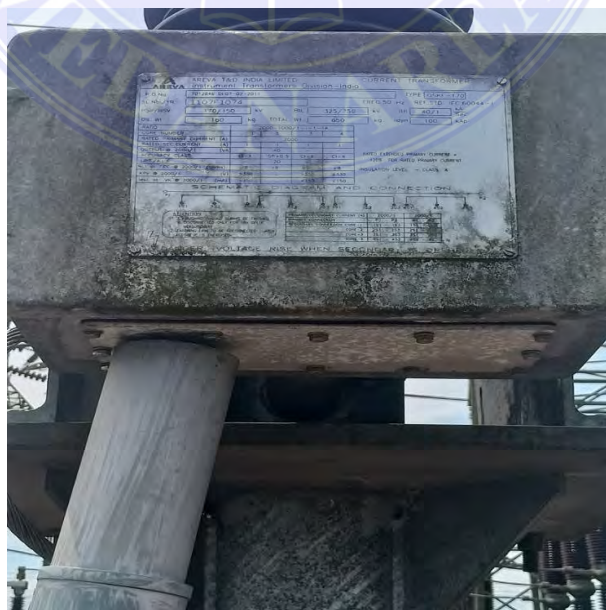
Gambar 4.4 Current Transformer (CT)
