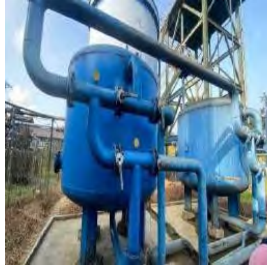
Gambar 3. 38 Pressure Sand Filter
