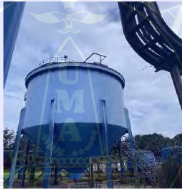
Gambar 3. 36 Water Clarifier Tank
