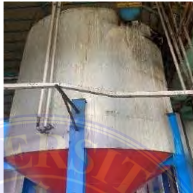
Gambar 3. 19 Continuous Oil Tank
