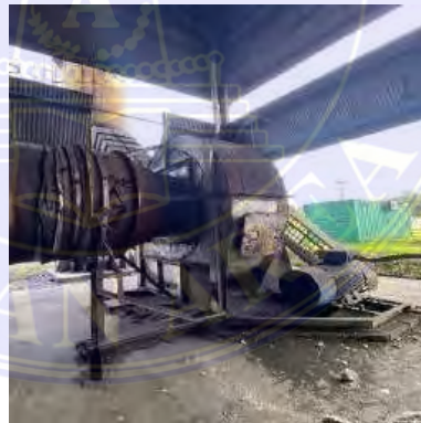
Gambar 3. 46 Induced Draft Fan
