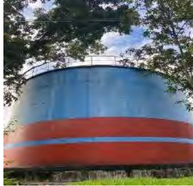
Gambar 3. 22 Oil Storage Tank
