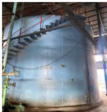
Gambar 3. 43 Feed Water Tank
