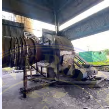
Gambar 3. 46 Induced Draft Fan
