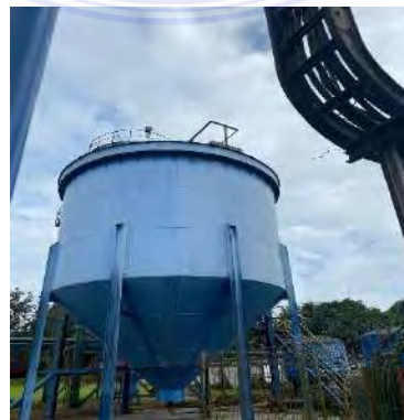
Gambar 3. 36 Water Clarifier Tank
