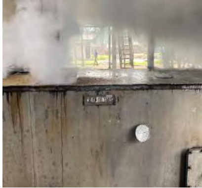
Gambar 3. 18 Crude Oil Tank
