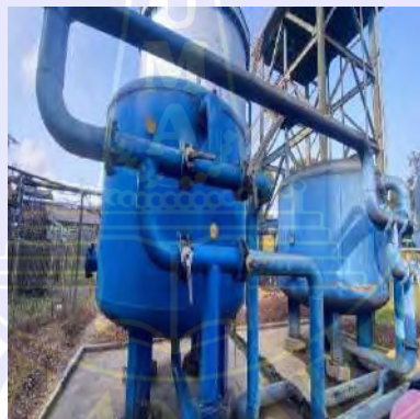
Gambar 3. 38 Pressure Sand Filter
