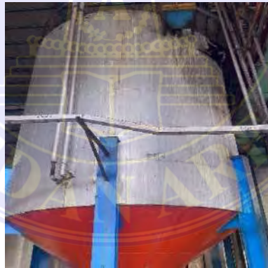
Gambar 3. 19 Continue Oil Tank
