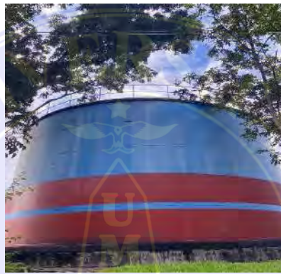
Gambar 3. 22 Oil Storage Tank
