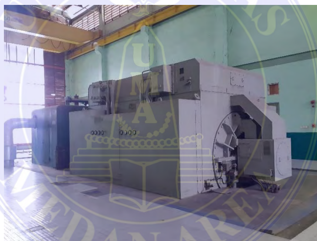
Gambar 2.1 Generator PT. Toba Pulp Lestari
