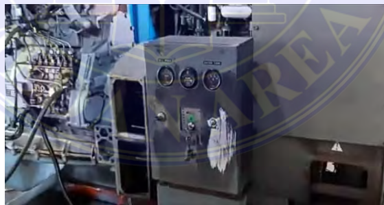
Gambar 3. 5 Panel pengontrol genset
