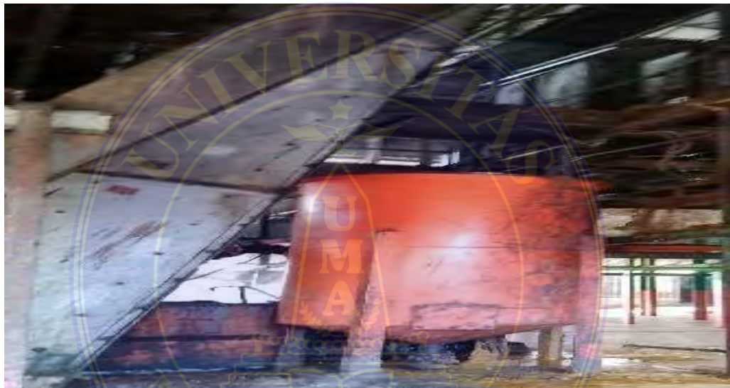
Gambar 3.13 Sand Trap Tank
