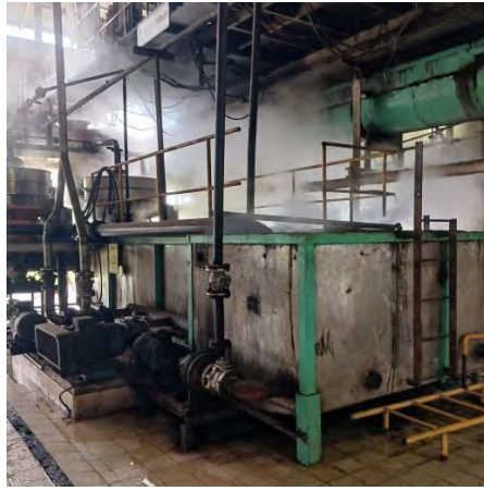
Gambar 3. 12 Crude Oil Tank ( Bak RO)
