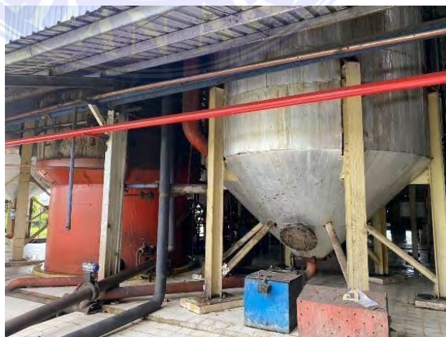
Gambar 3. 14 Continuous Settling Tank (CST)
