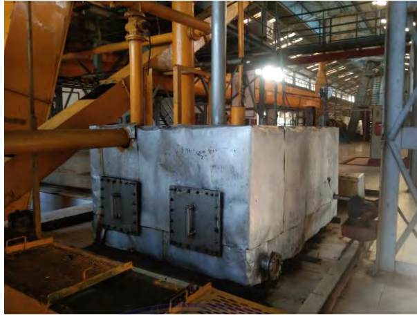
Gambar 3.16. Crude Oil Tank
