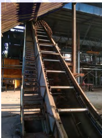
Gambar 3.4. Inclined Scrapper Conveyor
