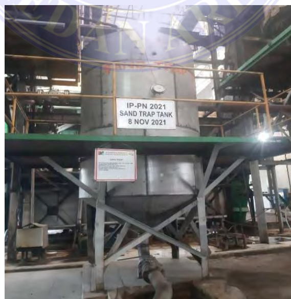
Gambar 3.25. Sand Trap Tank
