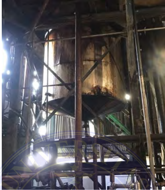
Gambar 3.27. Crude Oil Tank
