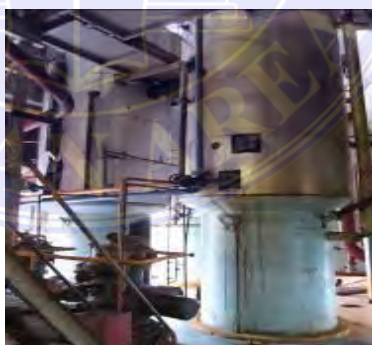
Gambar 35. Clean Oil Tank
