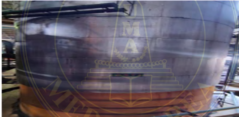
Gambar 3. 43 Continous Settling Tank
