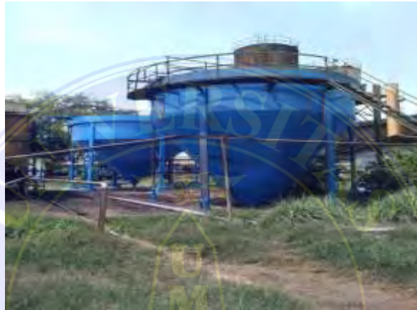
Gambar 3.31. Tangki Pengendapan ( Clarifier tank )
