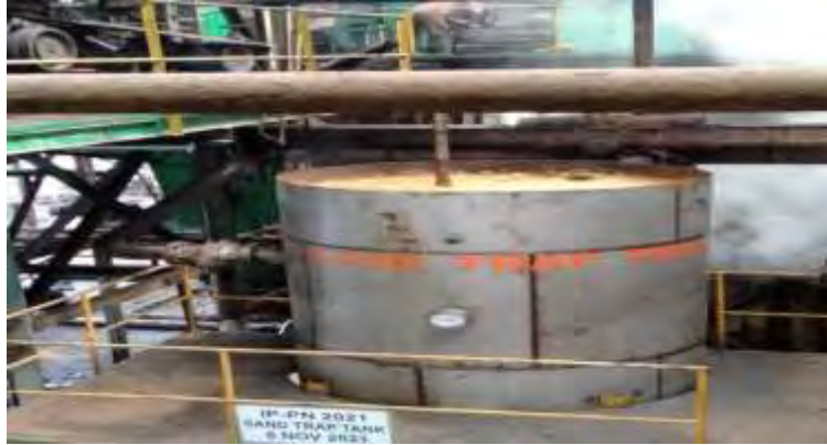
Gambar 3.13. Sand Trap Tank
