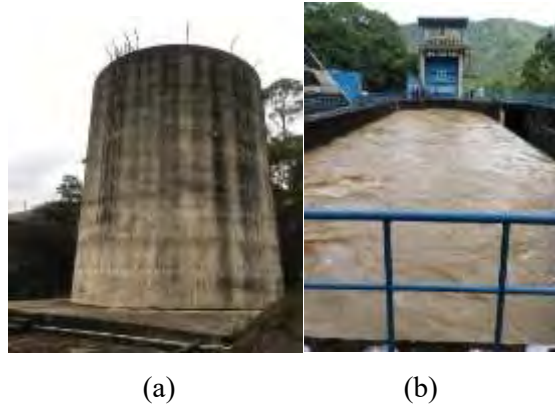
Gambar 3.6. (a). Surge tank , (b). Head tank
