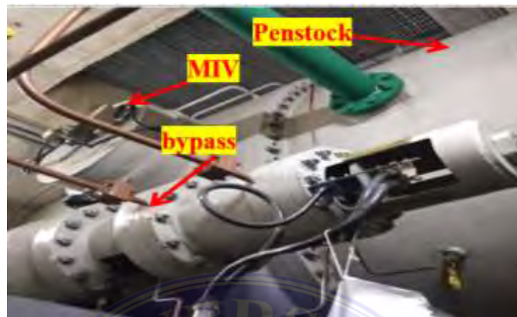
Gambar 3.8. Main inlet valve
