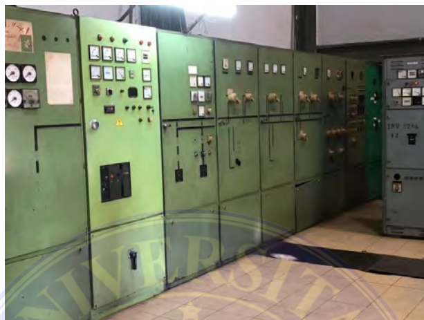
Gambar 3. 36 Panel Distribusi Tenaga Listrik
