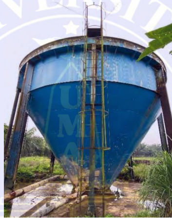
Gambar 3. 33 Fedd Water Tank
