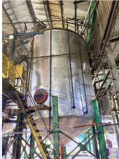
Gambar 3. 16 Continus Settling Tank (CST)
