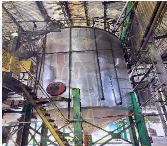
Gambar 3. 13 Continous Settling Tank (CST)
