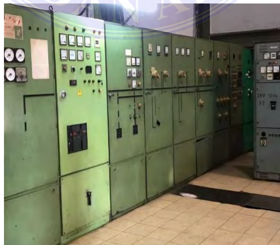
Gambar 3. 33 Panel Distribusi Tenaga Listrik
