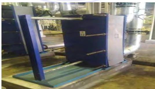
Gambar 3.5 Plate Heat Exchanger
