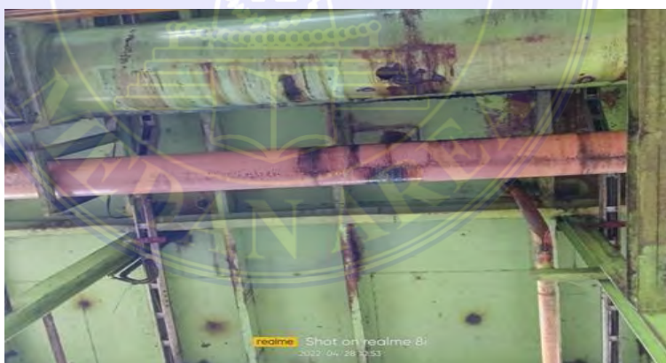
Gambar 3.29. Crude Oil Gutter
