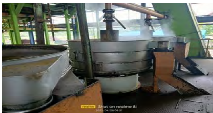
Gambar 3.30. Oil Vibre Separator
