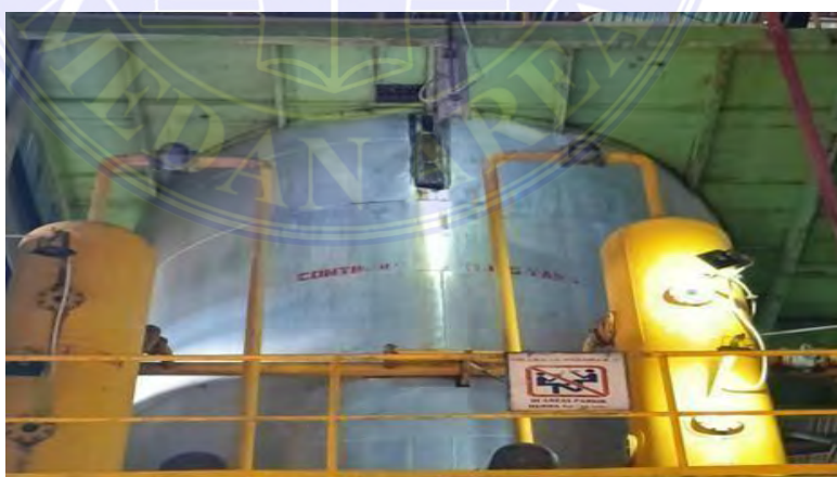
Gambar 3.31. Continious Settling Tank
